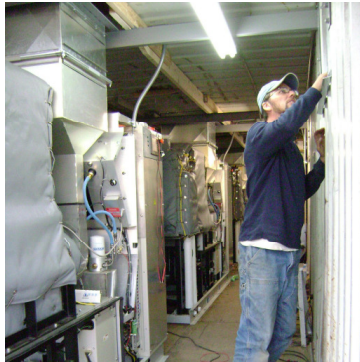
Preon Electrical Engineer assembling power equipment prior to final commissioning at a site near Vernal Utah
