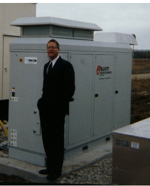
Preon CEO, Tim Tawoda, standing in front of an Elliott/Capstone TA100 micro-turbine at Savanna Depot.
