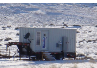
Dual TA100 at 5,000 feet elevation in Power River Basin near Gillette Wyoming. This module was designed and built by Preon's office in Sheridan Wyoming.
