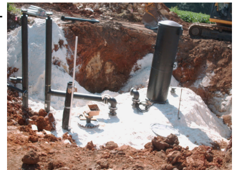
Biogas manifold at Monroe County landfill—Preon received an LOI in July 2010. Phase 2 will be the first bio-catalyst gas project.
